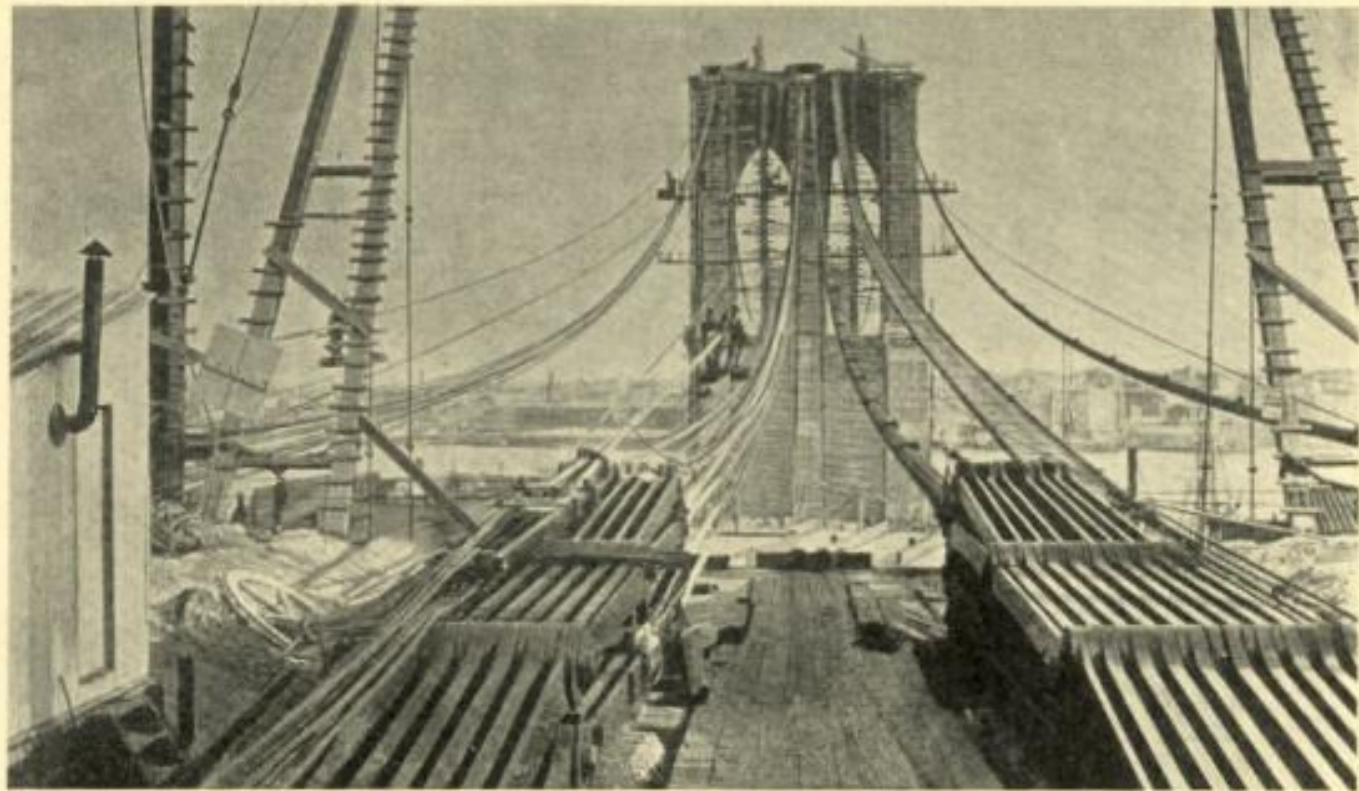
Brooklyn Bridge. Wire cables under construction. Last cable wire was run October 5, 1878.
